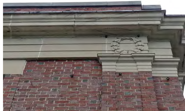
Open joints at sandstone entablature.
