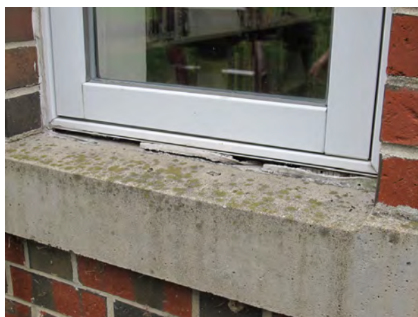
Deteriorated window caulking at 1989 addition.
