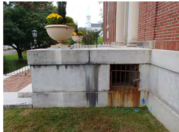
Ferrous staining at granite cheek wall.
