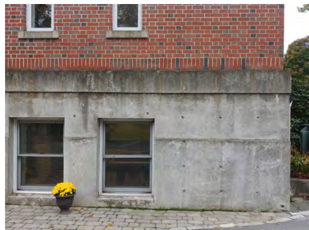
Unfilled snap-tie openings at concrete foundation wall. Staining at water table and wall.
