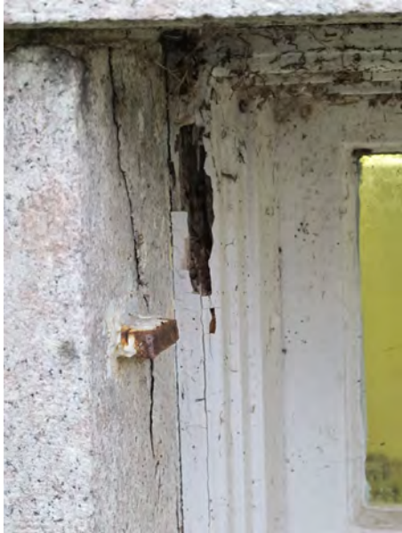
Damaged wood window frame and embedded steel pintle fragment.
