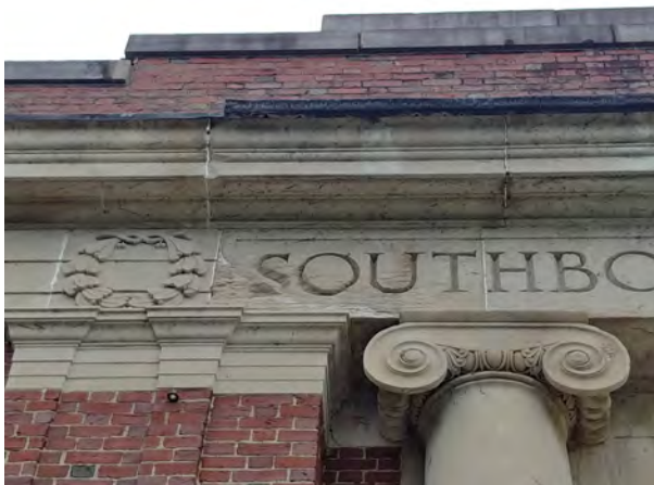
Eroded stone slab at south elevation containing incised lettering.
