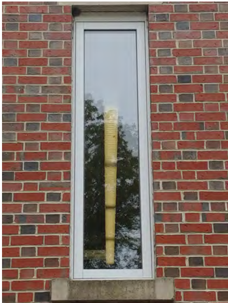
Perimeter sealants at 1989 windows are failing and need replacement.
