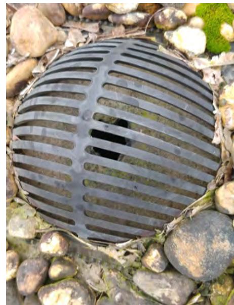
Restricted roof drain pipe opening.
