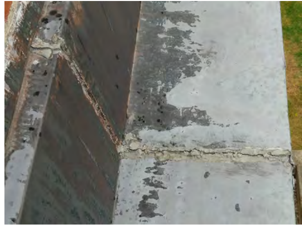
Cracked flashing solder joints.
