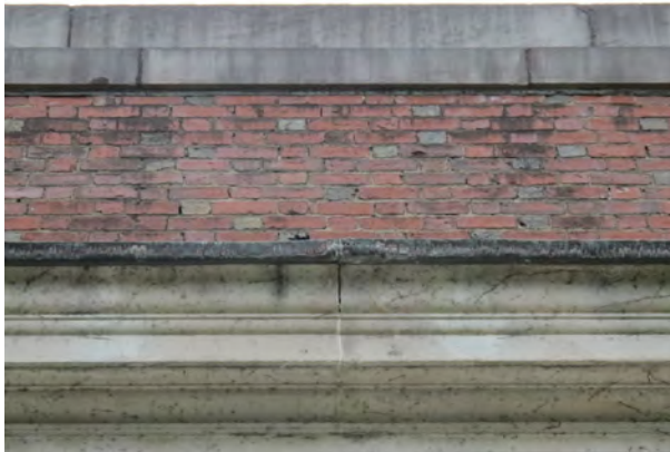
Failed mortar joints at brick parapet above south main entry stair.
