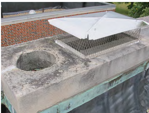
Uncapped chimney flue at parapet.
