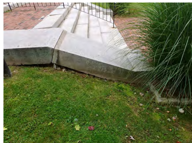
Shifted granite cheek wall at front entry.
