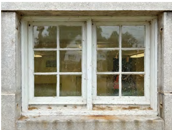
Failed paint coating at basement window, lack of exterior storm windows.
