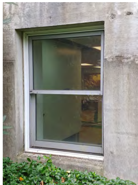
Deteriorated window sash at ground level of 1989 addition.
