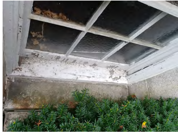
Deteriorated window sill at ground level, east elevation.
