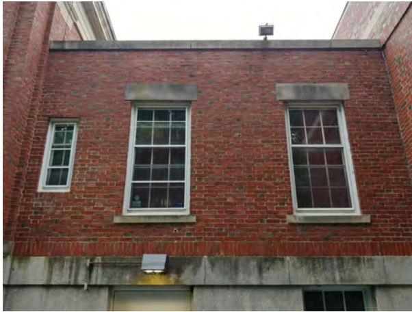
Staining of foundation at east elevation of early addition.
