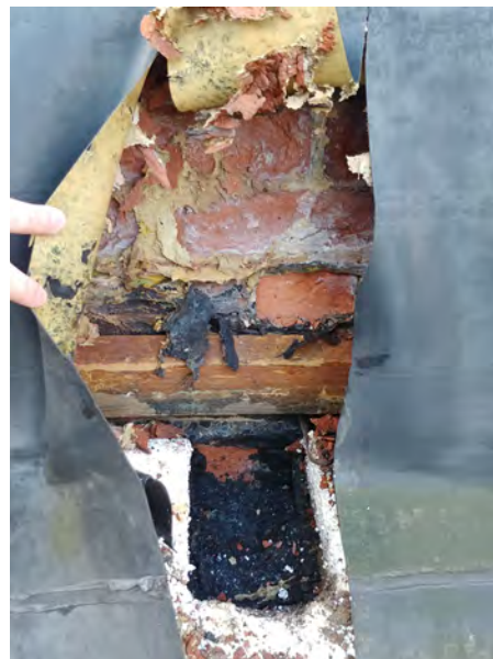
Saw cut inside north-facing parapet reveals extreme damage to masonry.
