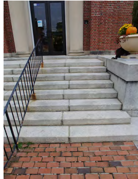
Granite stair slabs at south entry have shifted and pavers show mortar loss.
