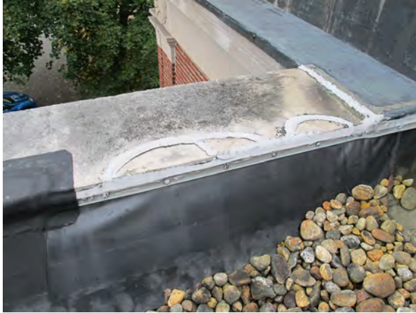
Spalled stone coping at parapet due to improperly installed termination bars.
