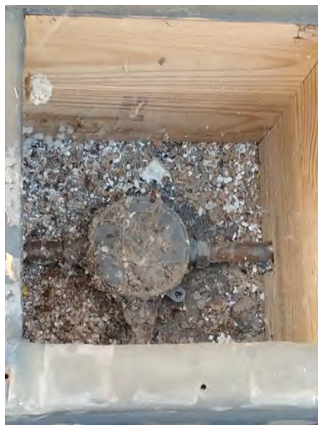
Saw cut. Three wood boxes protect electrical junction boxes above original 1912 chandeliers below.
