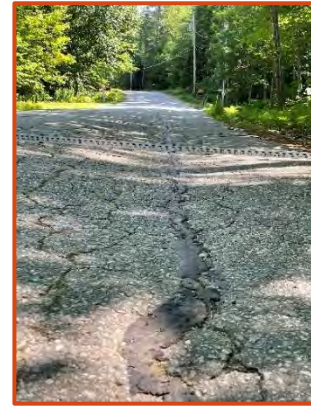
Hebron RSMS - Rutting on Bear Mountain Road
