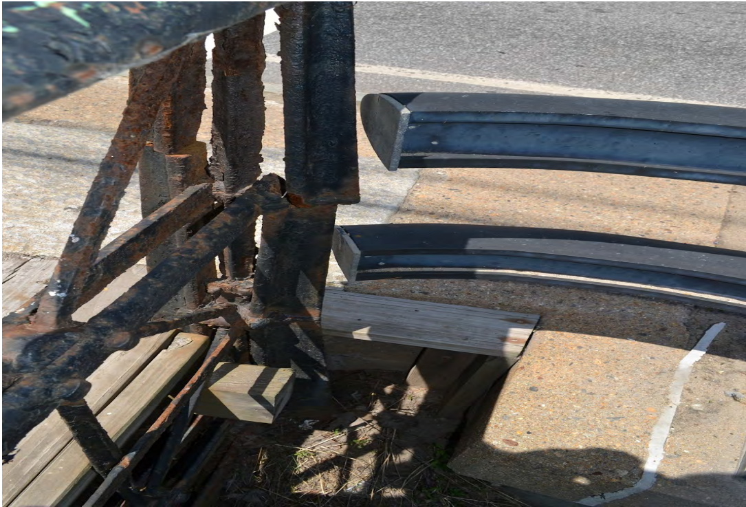
Corroded and Cracked Cast Iron End Post
