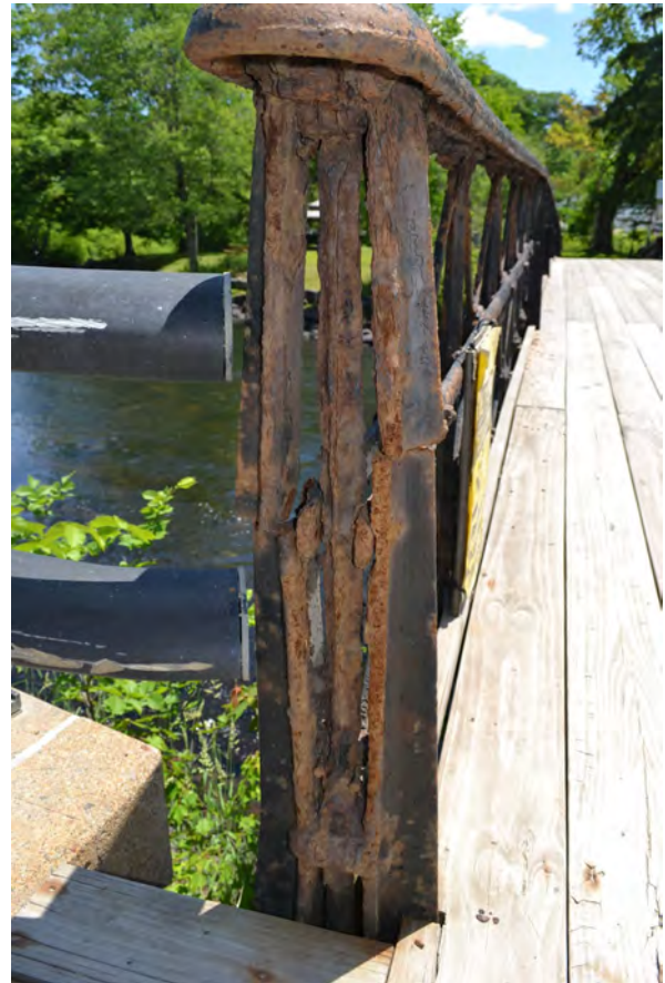
Corroded and Cracked End Post
