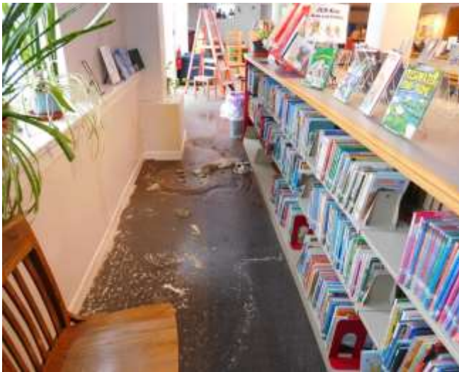
A steam valve burst in our Children's Room in 2016
