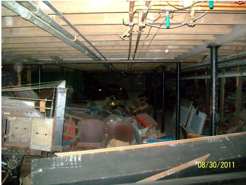
View of waste located in basement #3 of building #2
