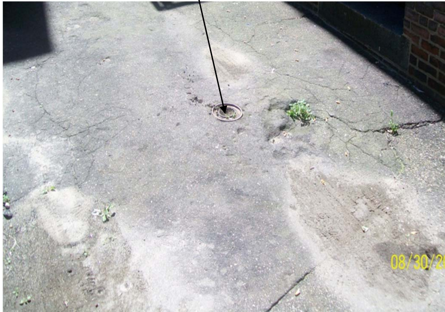
Location of reported UST and associated former fill port in the alcove along the Canal Street portion of the subject property
