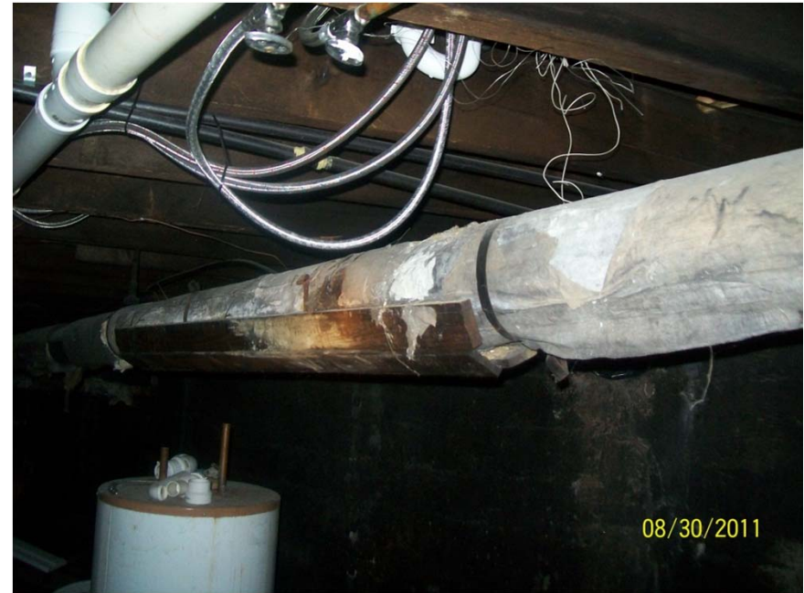
View of suspect asbestos containing pipe insulation located above the gas-fired furnace in basement #1 of building #1
