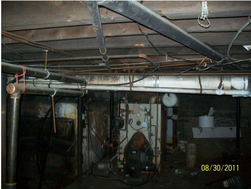
View of oil-fired furnace and former boiler located in basement #3 of building #2
