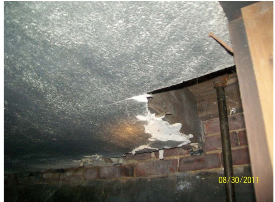
View of suspect asbestos containing materials located above the furnaces in basement #3 of building #2
