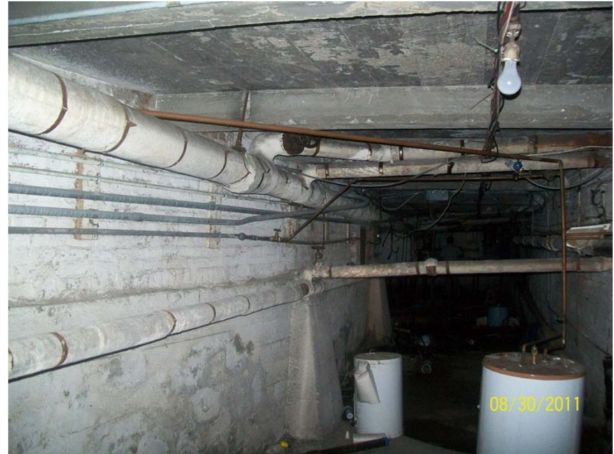
View of the suspect asbestos containing materials in the basement area known as the "heat and fresh air chamber" located under building #2
