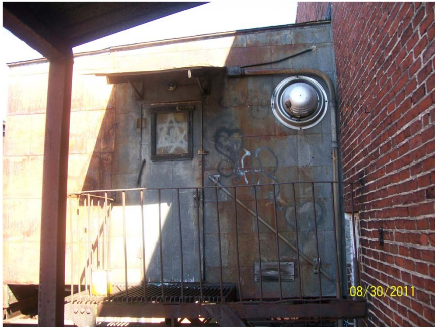
View of the projector room located in the courtyard between buildings #1 and #2
