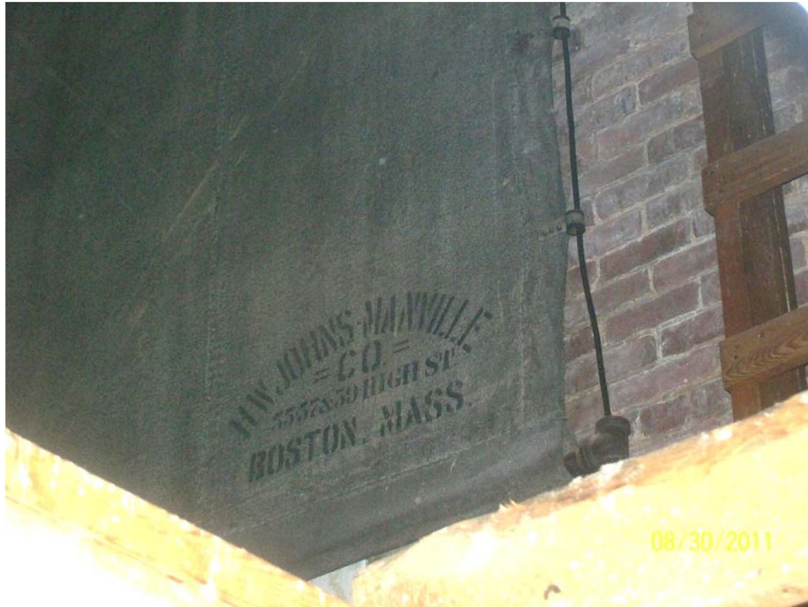
Close-up view of suspect asbestos curtain located in building #2
