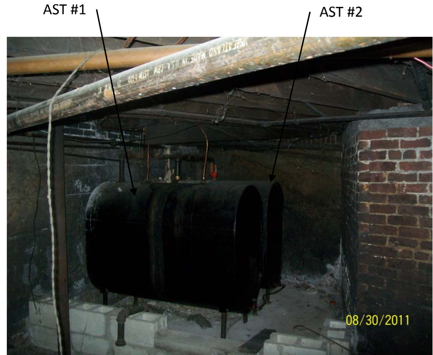
Two 275-gallon No. 2 fuel oil ASTs located in basement #3 of building #2
