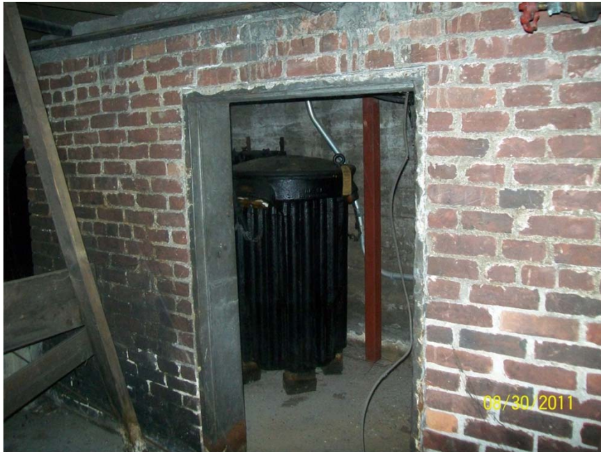
View of electrical transformer located in basement #3 of building #2
