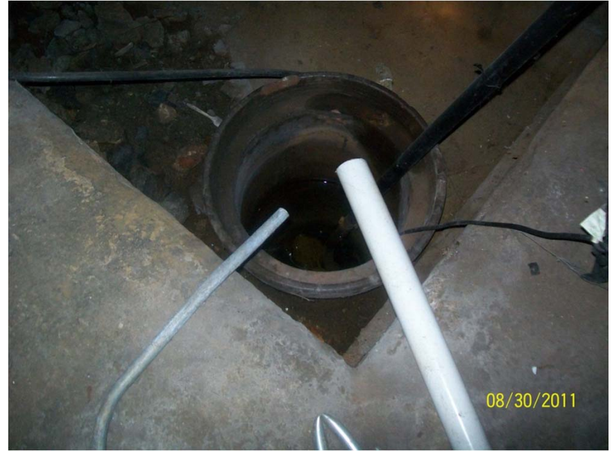
Water filled sump located in basement #3 of building #2
