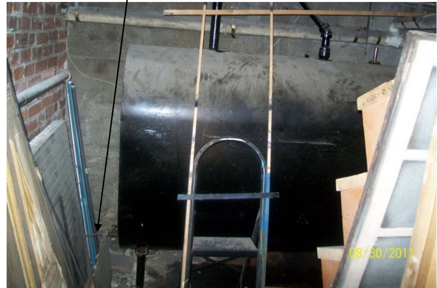
AST #3 located in basement #2 of building #2
