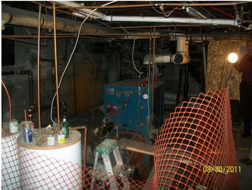
Gas-fired furnace and hot water tanks located in basement #1 of building #1
