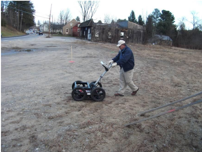
Picture 2 Representative view of the ground penetrating radar (GPR) survey by Dig Smart of Maine.
