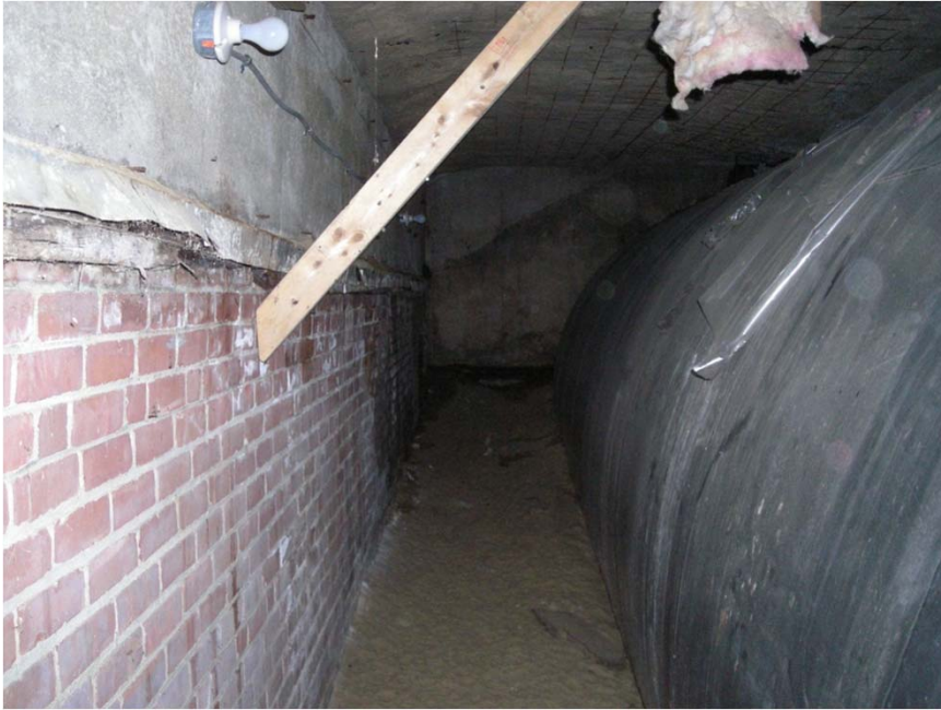
View of the east side of the Underground Storage Tank, as viewed from inside the UST building extension.
