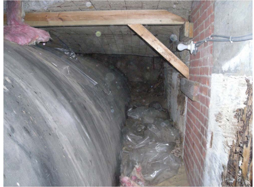
View of the west side of the Underground Storage Tank, as viewed from inside the UST building extension.
