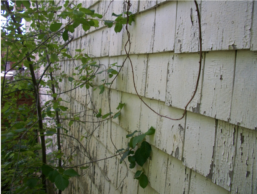
Picture 5 - View of peeling exterior Lead-Based Paint on western side of barn portion of garage/barn building
