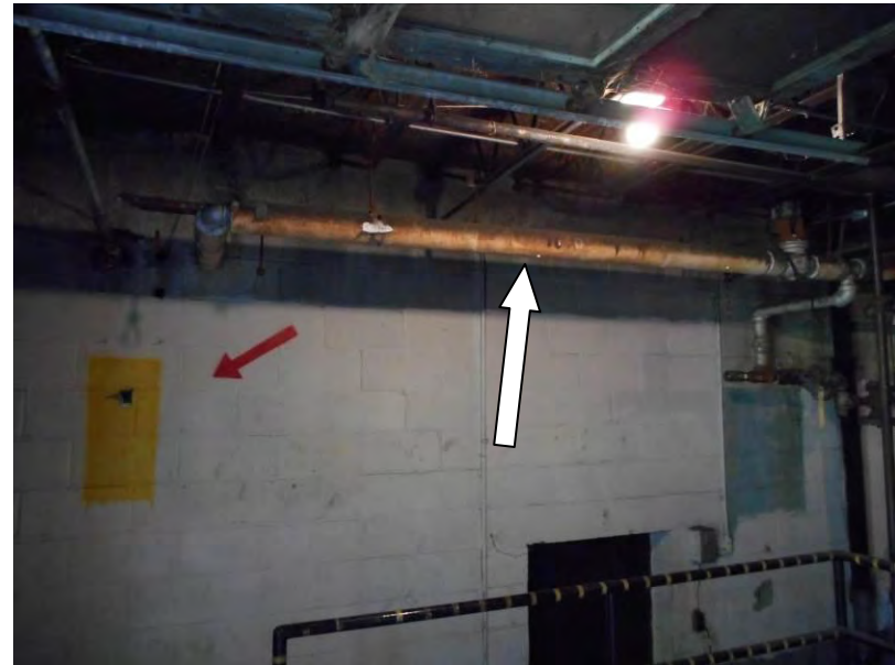
26. Representative photo of ACM TSI identified at the Site.
