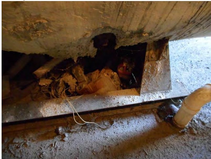
23. Representative photo of ACM TSI identified at the Site.
