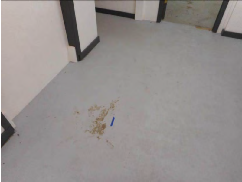
17. Location of CA-PCB-4 collected from upper layer of gray floor paint in the retail store. CA-PCB-1 collected from lower layer.
