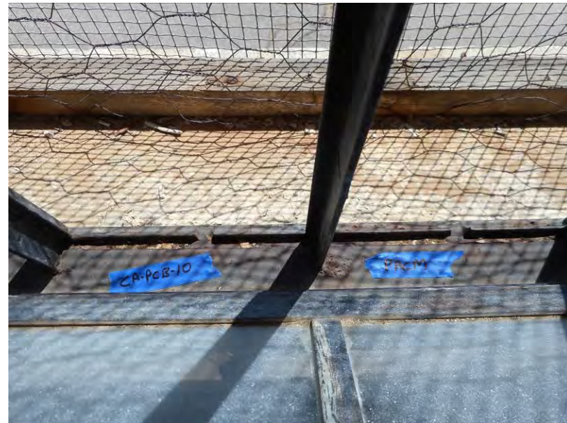
22. Location of CA-PCB-10 collected from window caulk in the lower building.
