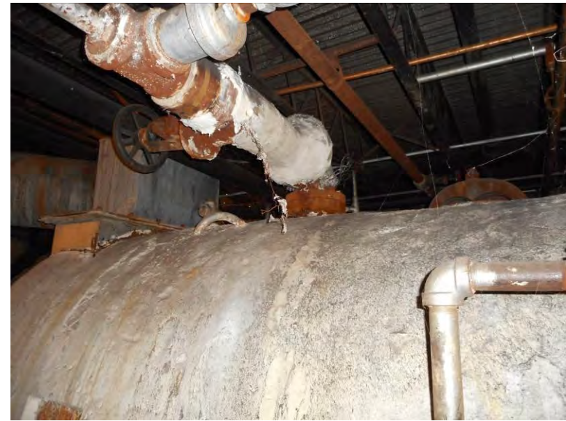
28. Representative photo of ACM TSI identified at the Site.
