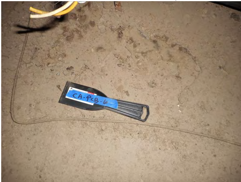
19. Location of CA-PCB-6/CA-PCB-DUP collected from gray floor paint in the boiler room of the two-story building.
