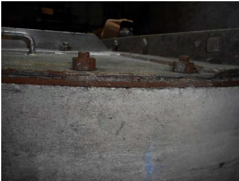
27. Representative photo of ACM gasket at the Site.
