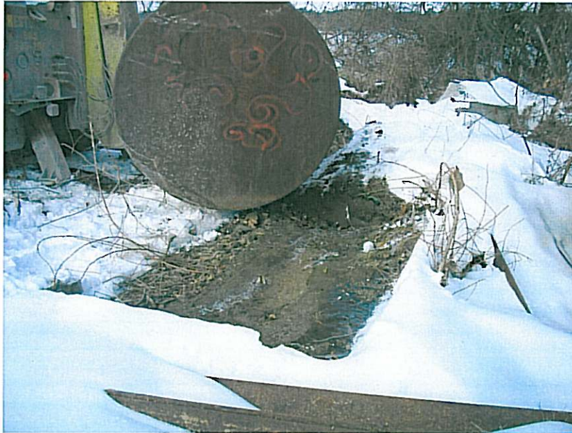
5. View looking to the west of the 1,500-gallon AST during removal activities on January 12, 2010.
