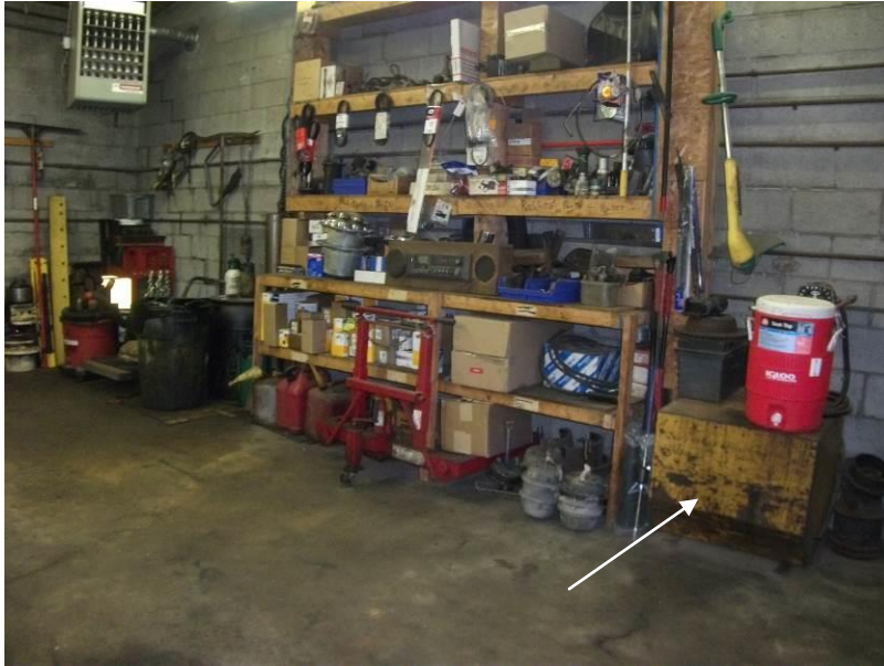
13. Southern garage bay area within Site building, note diesel tank in right side of photograph. Note the floor staining.
