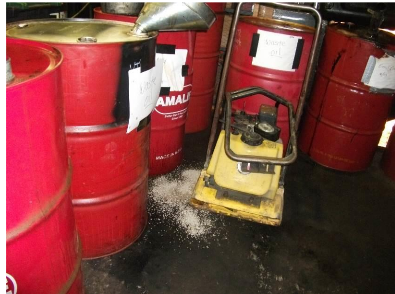
10. Evidence of spills in the drum storage area. Note the staining and absorbent material.
