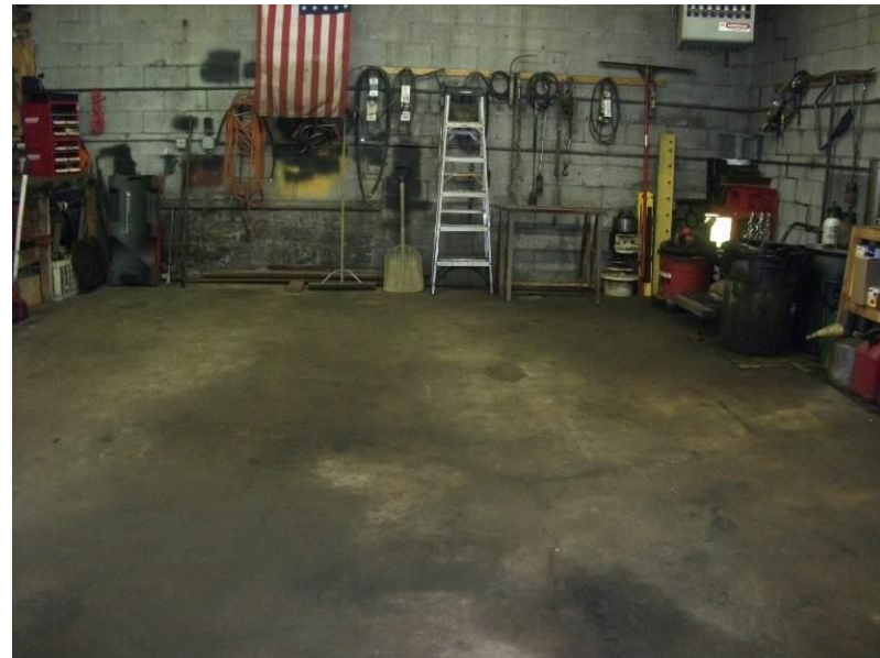
12. Southern garage bay area within Site building. Note the floor staining.
