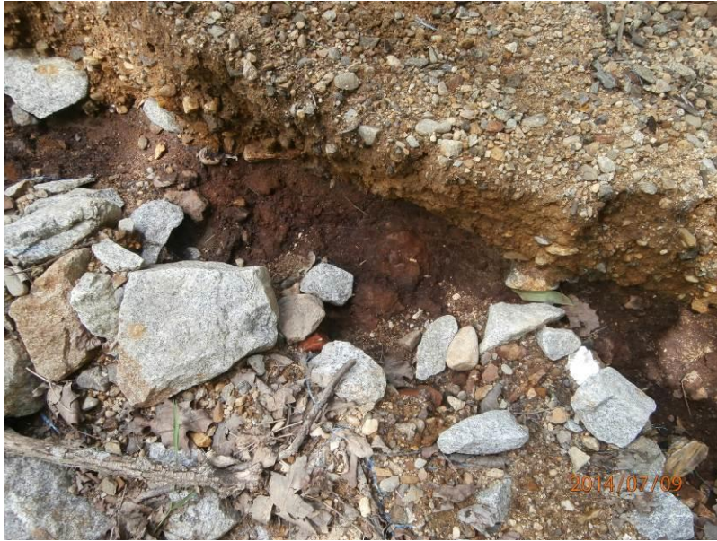
25. Image showing metal shaving fill to the southeast of the Site building as indicated by the rusty colored area.
