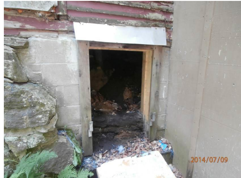
26. Image showing the crawl space with suspected ash fill beneath the Site building.
