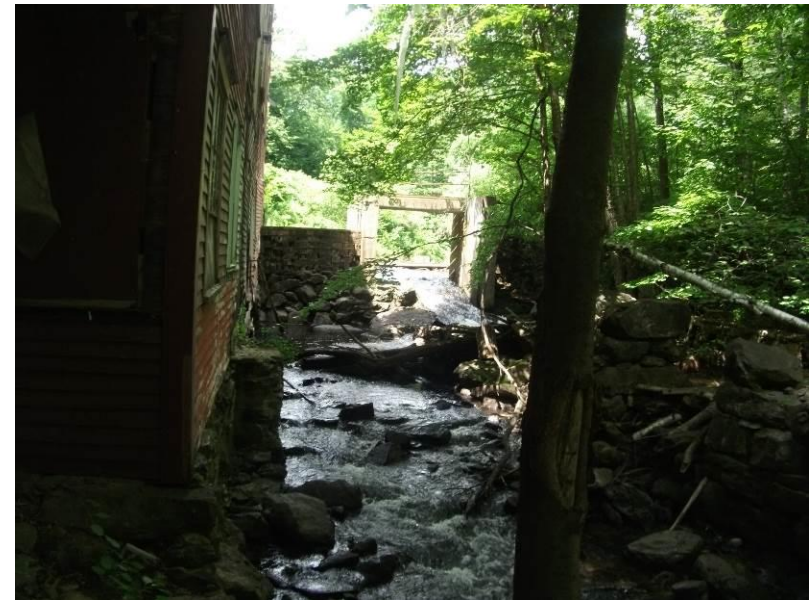
4. Image showing Chance Pond Brook flowing along the building foundation looking northwest.
