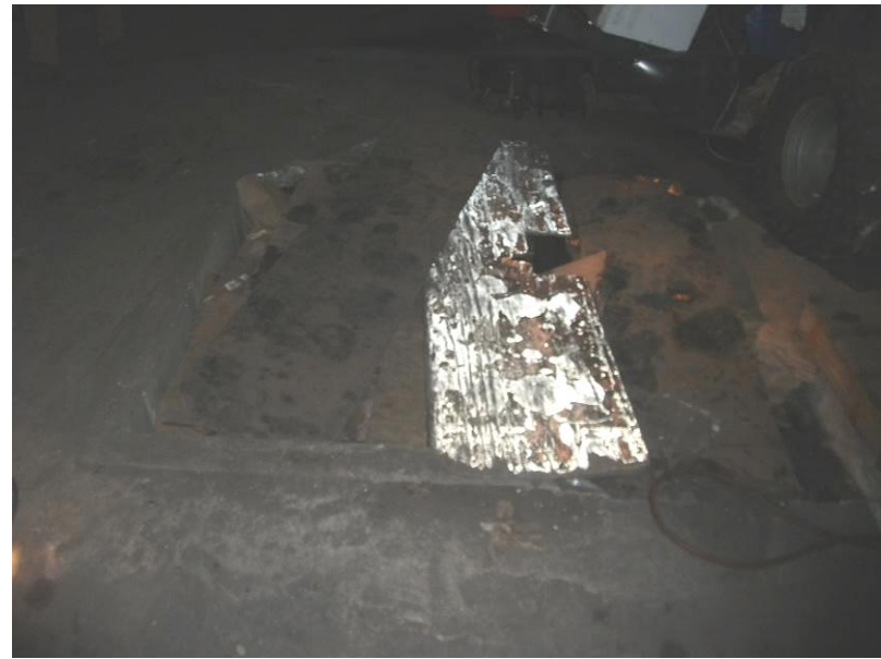
20. Image showing the sand shaker motor pit (filled with debris) and staining on floor around the pit.
