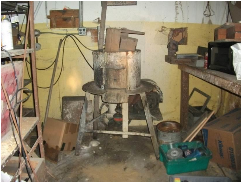
7. Image showing typical remnant equipment within the building. Note the floor staining.
