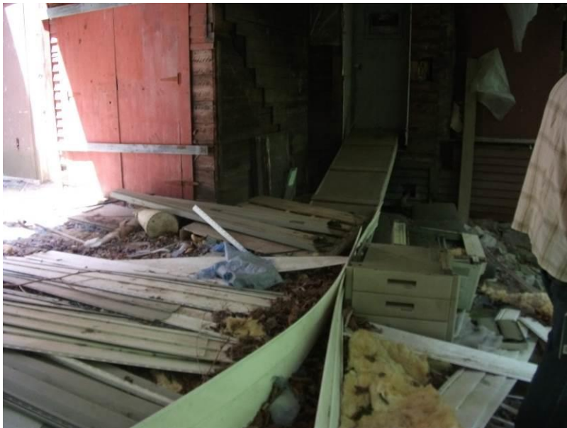
23. Image showing typical debris in exterior portions of the Site.
