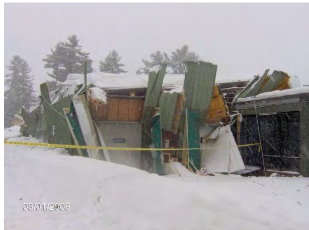
Figure 7: Roof collapse, Franklin, NH - 2008
