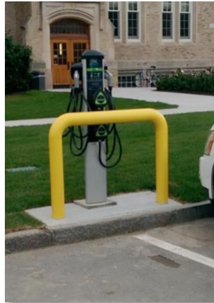
Figure 16: Tire stops used for EVSE protection (Source: Energetics)
