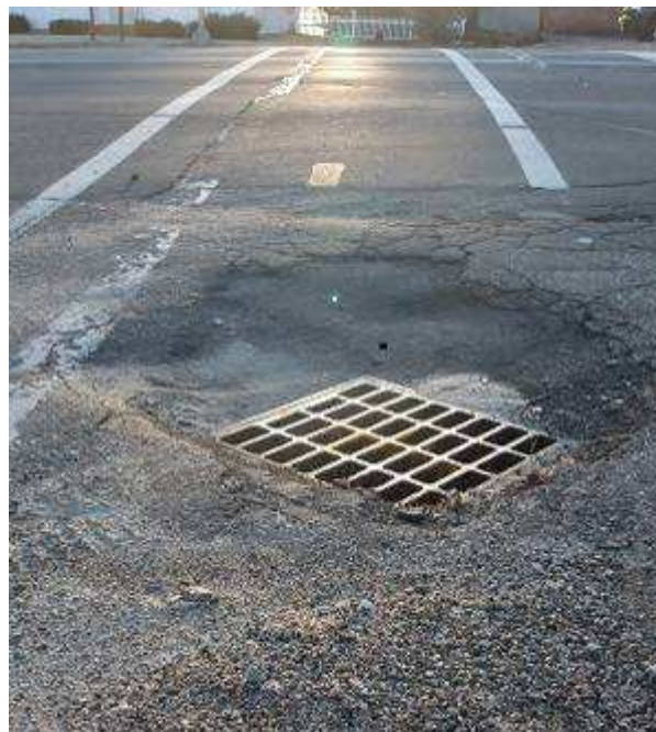
Fig. 22 – Storm drain and gravel in NH Route 25 crosswalk where safe sidewalk ramp should be located.
