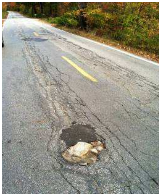
Fig. 17 - Failing pavement along NH 171 in Tuftonboro. Note the heaved cobble, longitudinal cracking, and lack of shoulder space along this route, which is identified as being part of the regional bicycle route system on the NH Regional Bicycle Map (LRPC photo)
