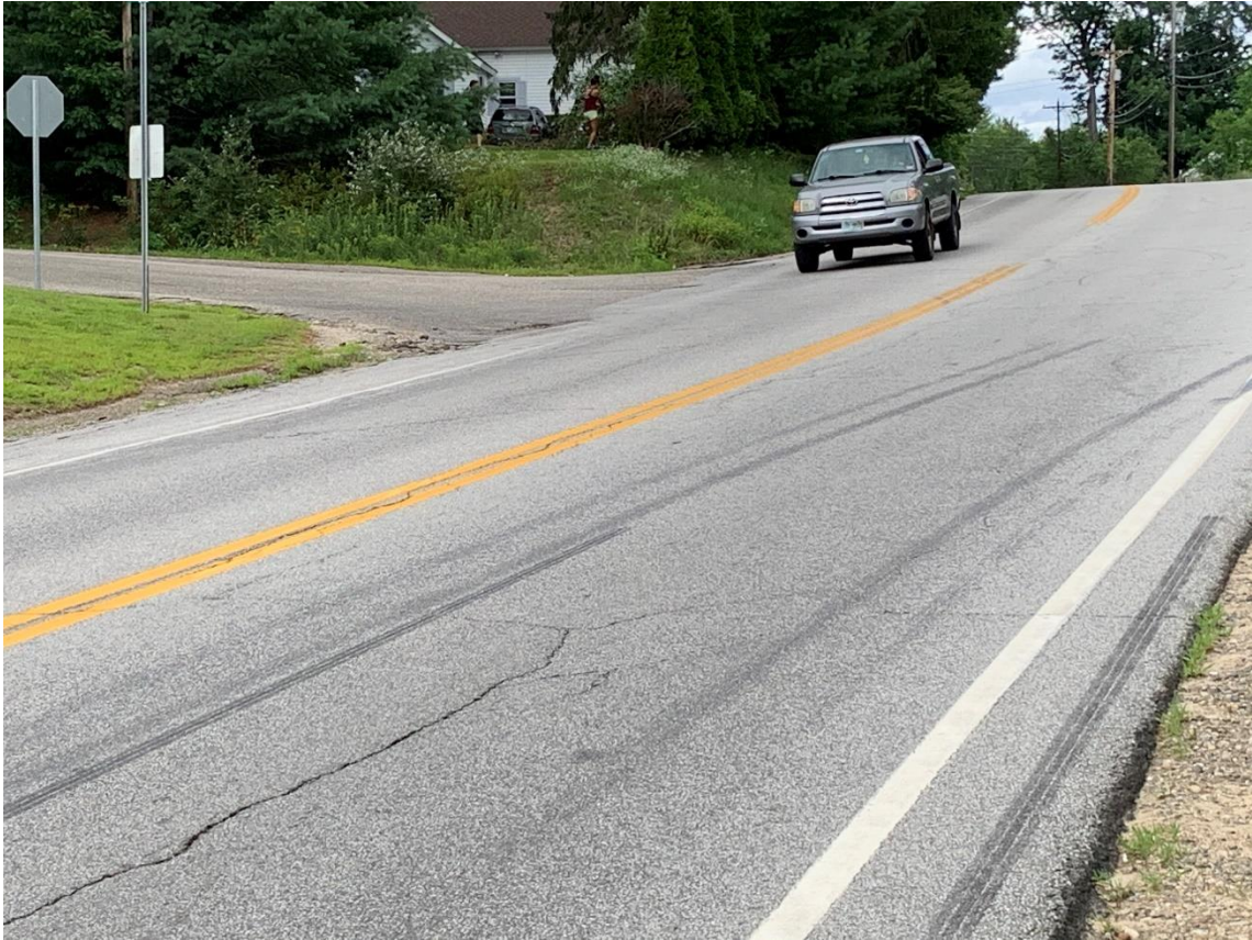
2-A NH Route 25/ True Road intersection facing west towards. Note inadequate shoulder
