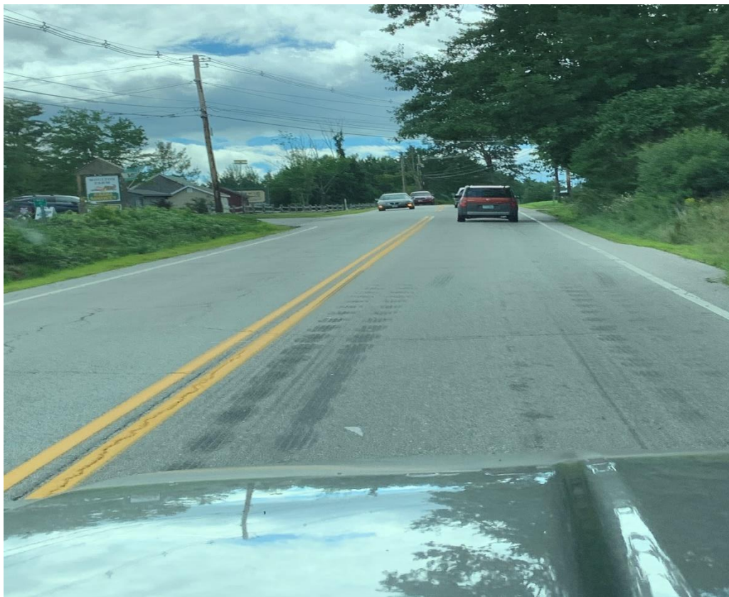
3-B NH Route 25 at Quarry Road facing west. Note inadequate shoulder.
