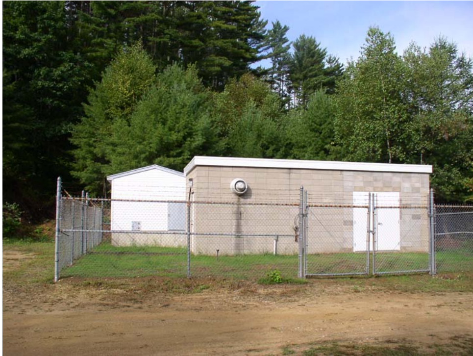
One of two pump stations for gravel packed wells providing the Belmont Public Water supply.
